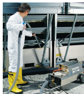
CTV-1501 Wet-vacuum tower floors without shut-downs.
